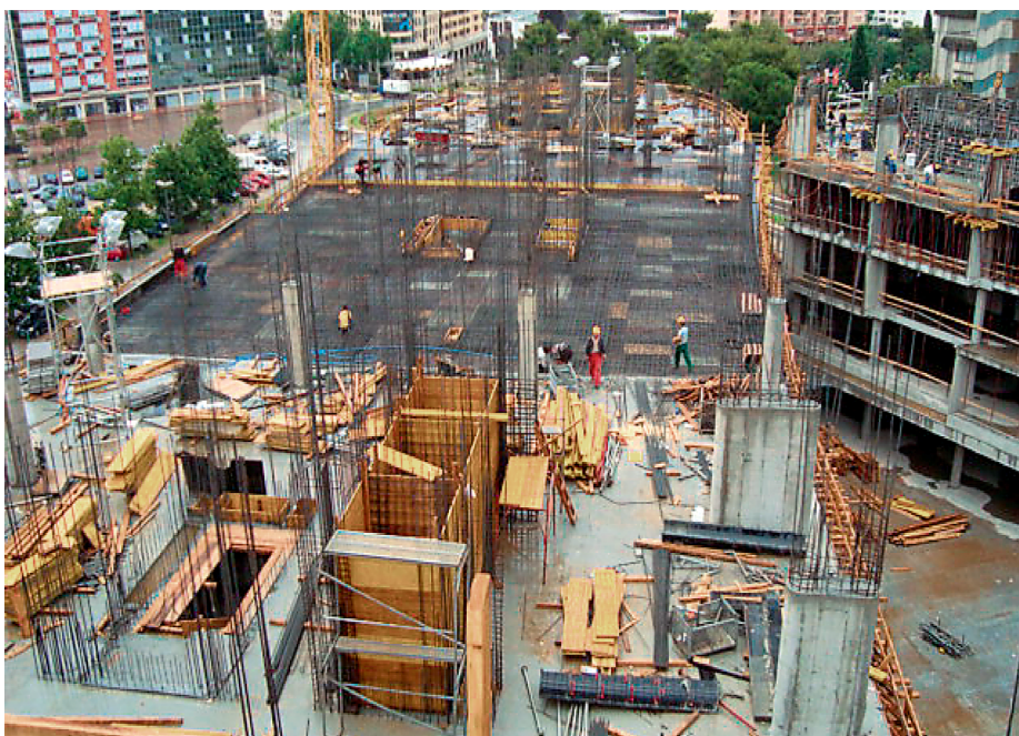
Figure 2: Works in progress on concrete blocks on the business part of ACC
